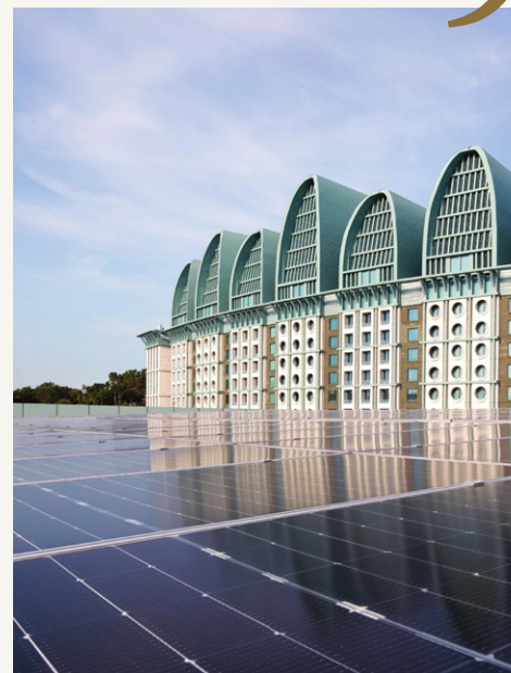
RWS rooftop solar panels
